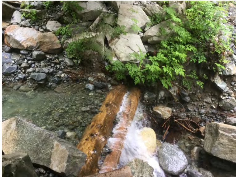
Riprap at both banks founded on organics
