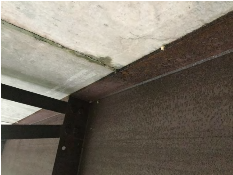
Corrosion noted at deck joints
