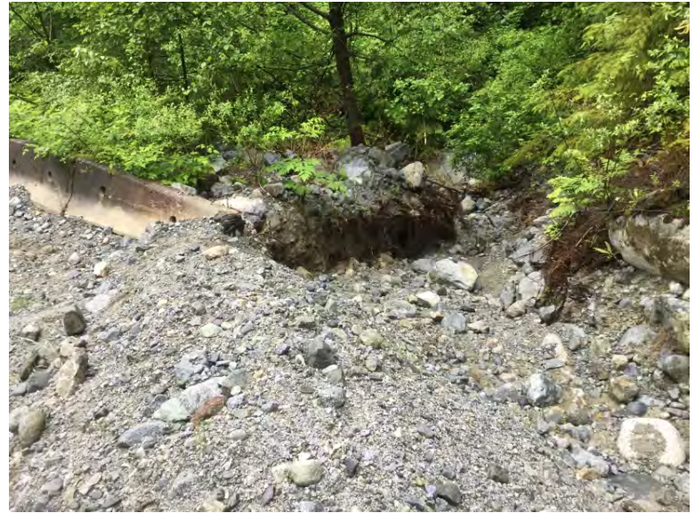
Upstream left approach ditch scour
