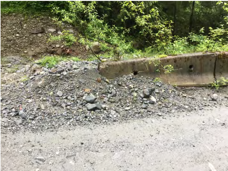
Missing both bull noses at left approach
