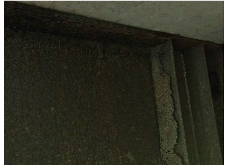
Corrosion noted at right bank
